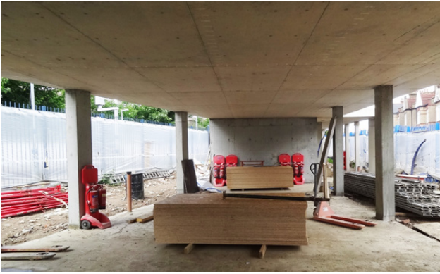
Commercial Development, Formwork and Concrete construction by our company for a Developer in South East London exposing our company skills
